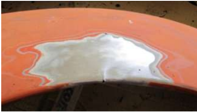
347. Crack, Front side - Before
